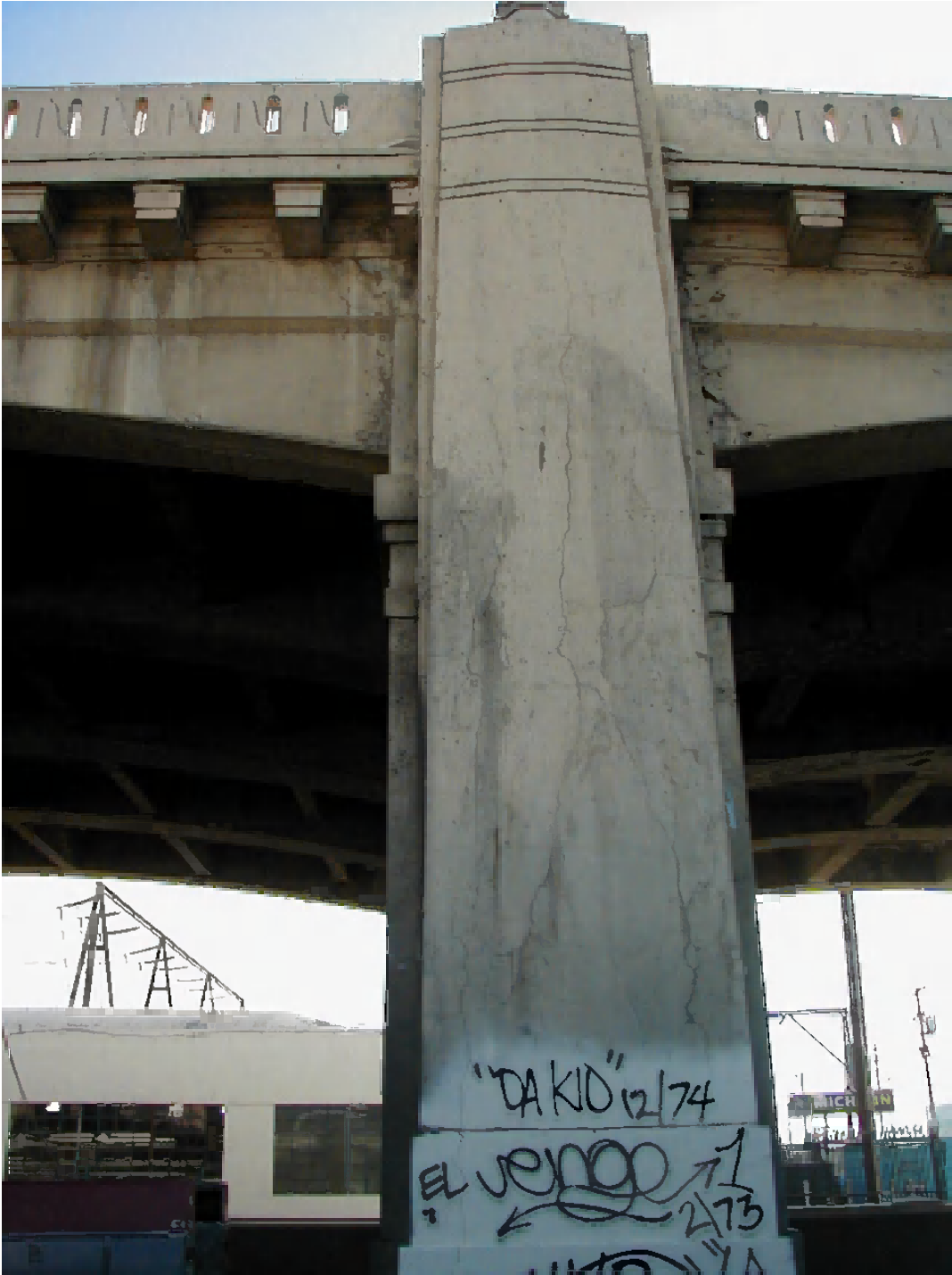
Figure 5: Typical cracking on outside face of column.
