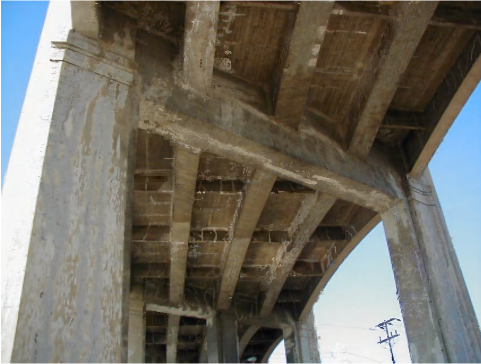
Figure 8: Typical cracking pattern in bent cap and girders.
