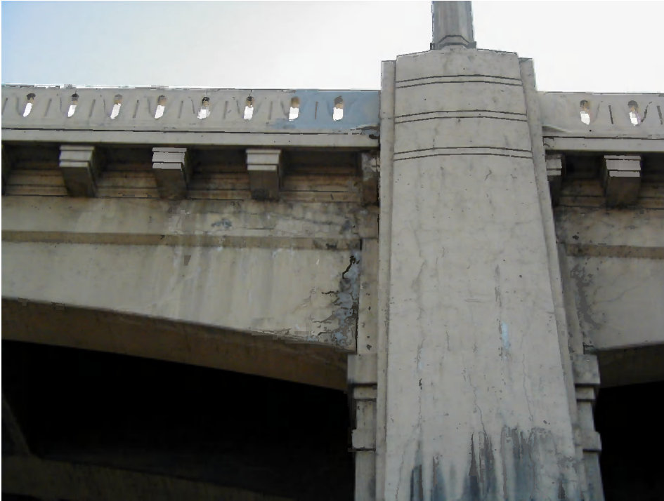
Figure 10: Peeling paint and longitudinal web cracking in girders.
