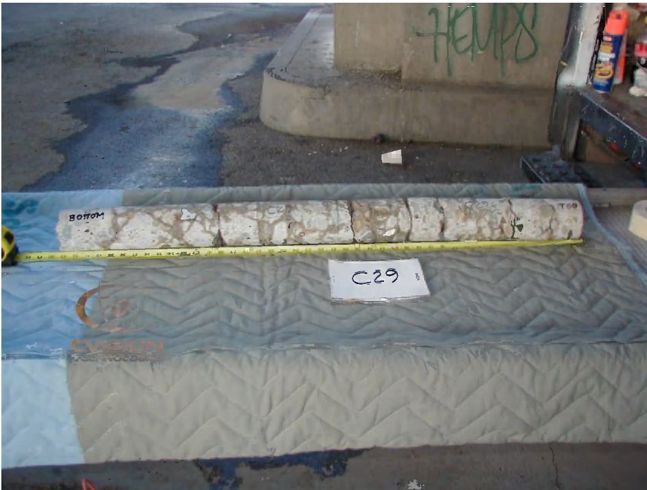
Figure 19: Severely cracked core that had 6 breaks when removed from a column.
