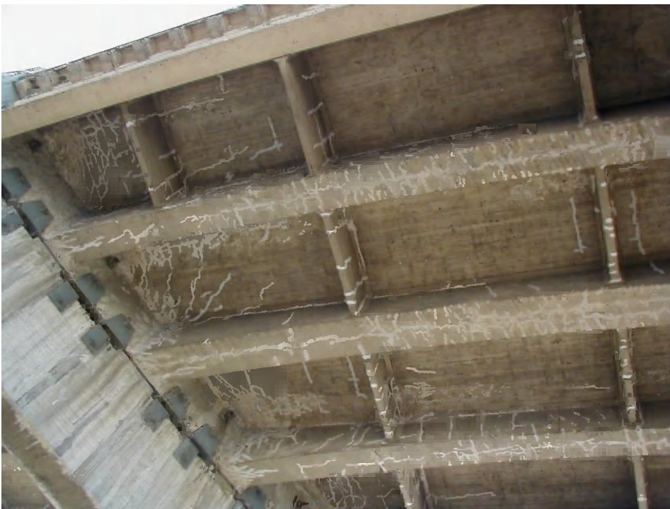
Figure 9: Typical crack patterns noted in girders.
