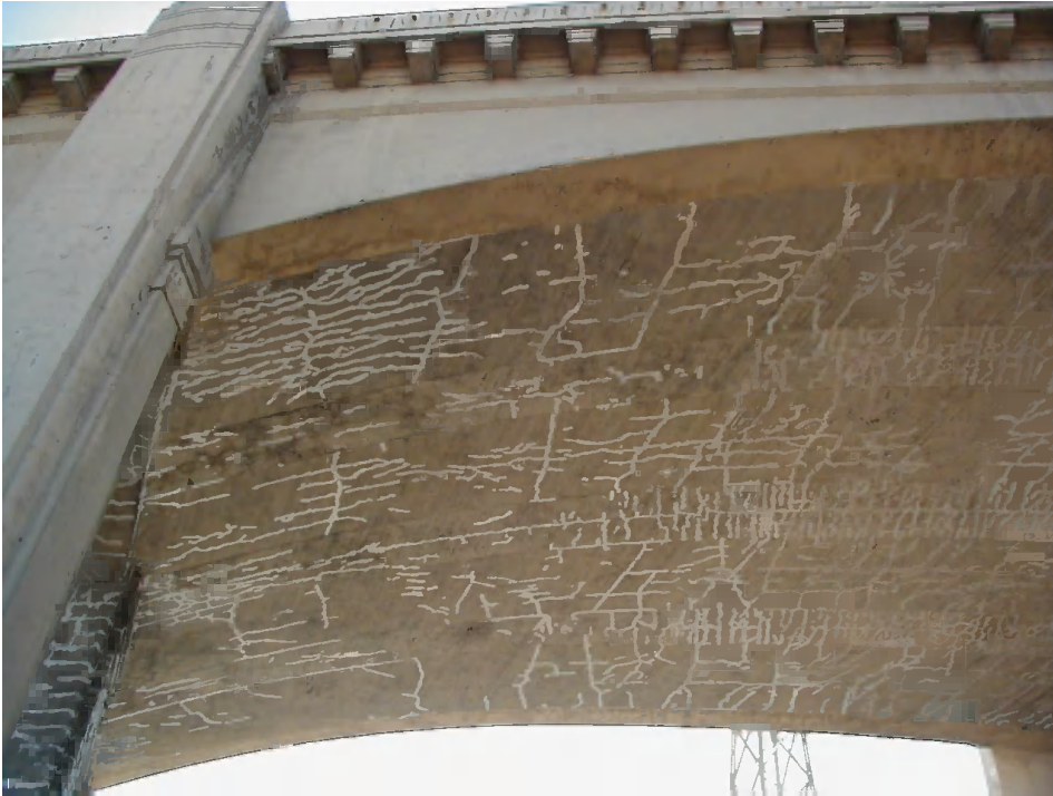
Figure 14: Map cracking in the infill soffit of girders at bays over railroad tracks.
