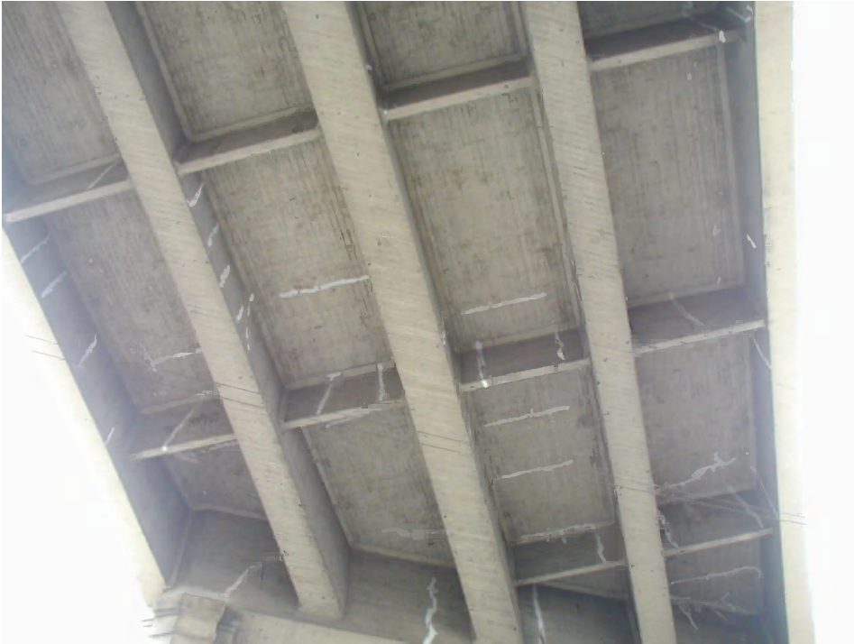
Figure 12: Typical crack pattern on deck and girder at lightly distressed locations at the east end
