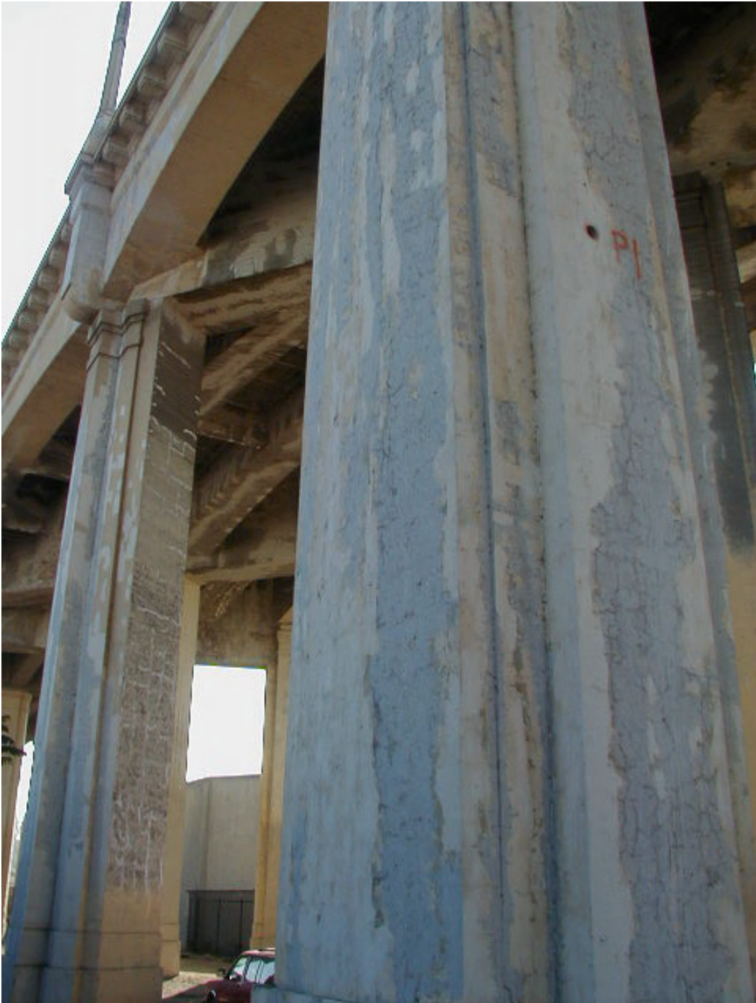
Figure 6: Typical condition of columns at east end of bridge.
