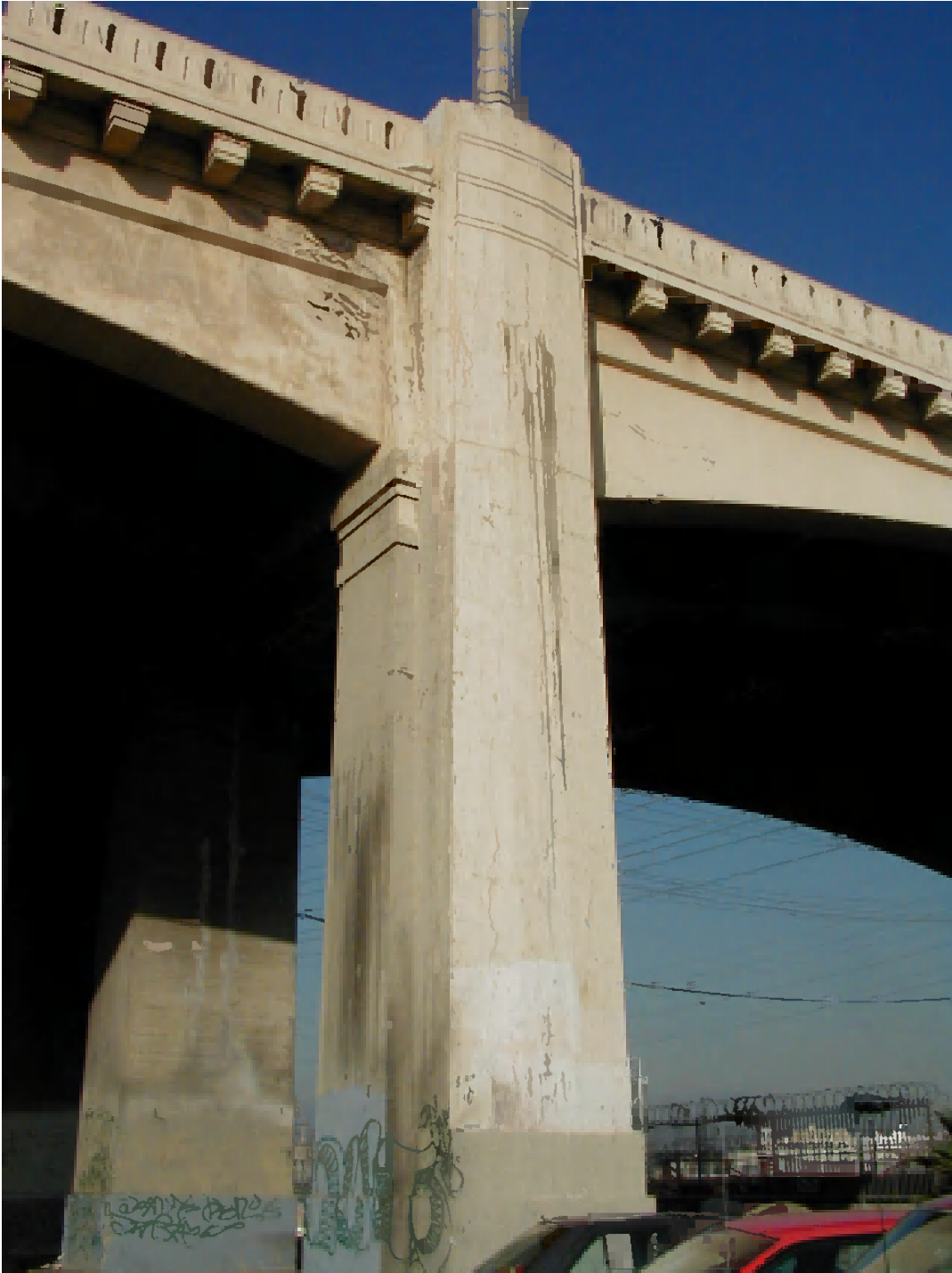
Figure 7: Typical horizontal crack in column at level of bent cap.
