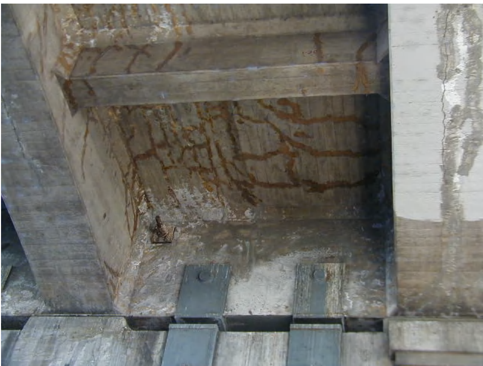
Figure 13: Dense map cracking in deck soffit at bent cap.
