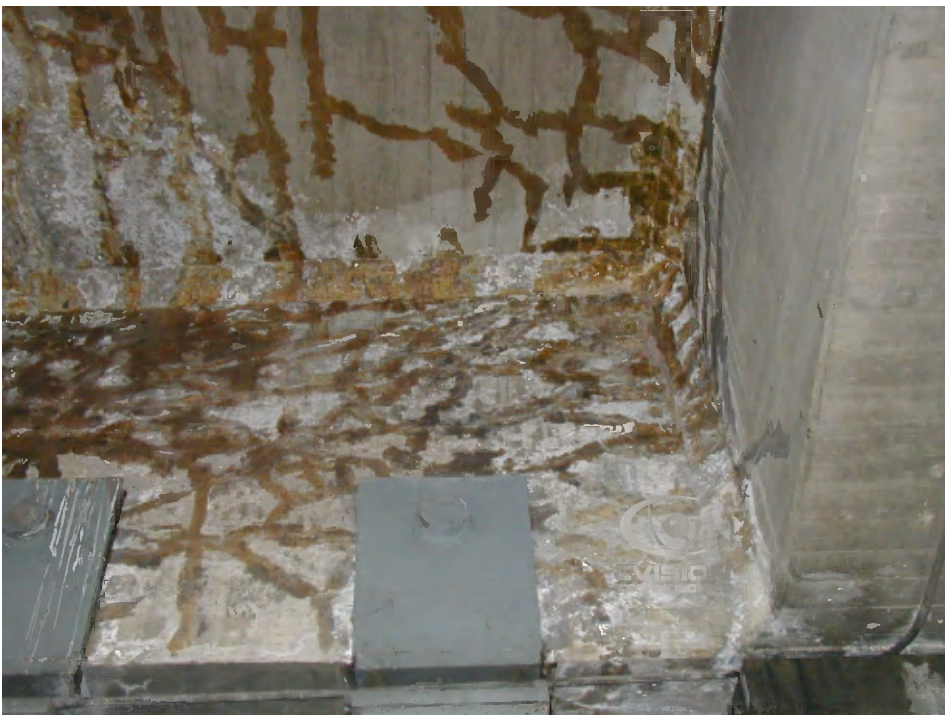
Figure 11: Severe cracking in bent cap and deck soffit. Note the efflorescence in the deck.
