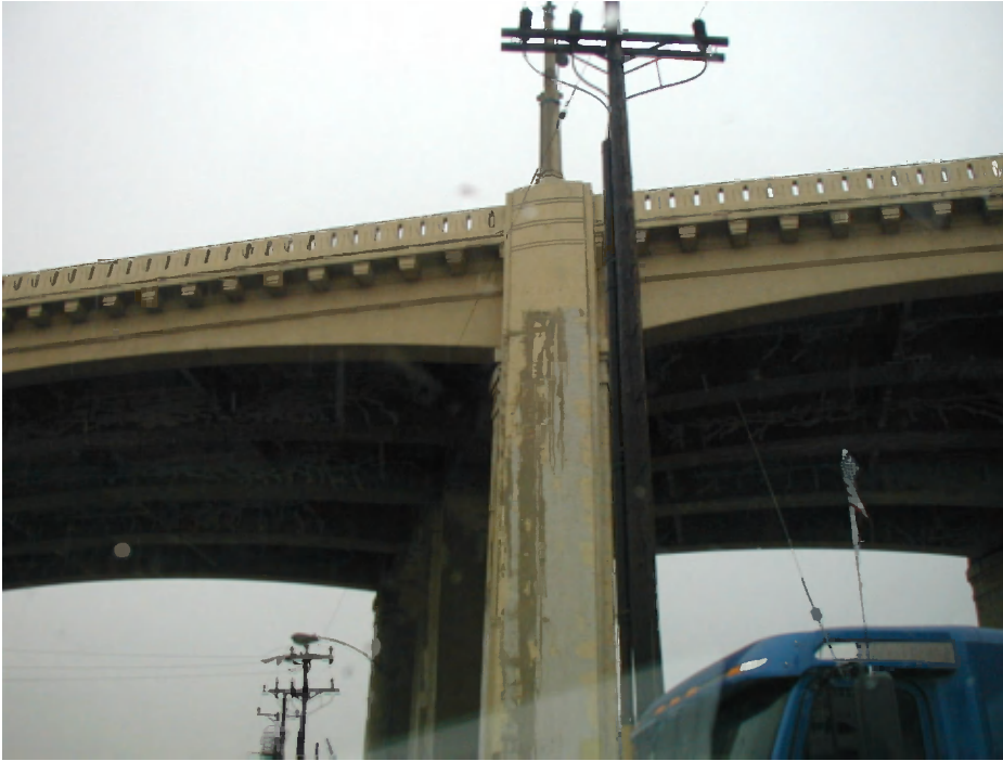
Figure 26: Water leaking from a typical horizontal column crack at bent cap.
