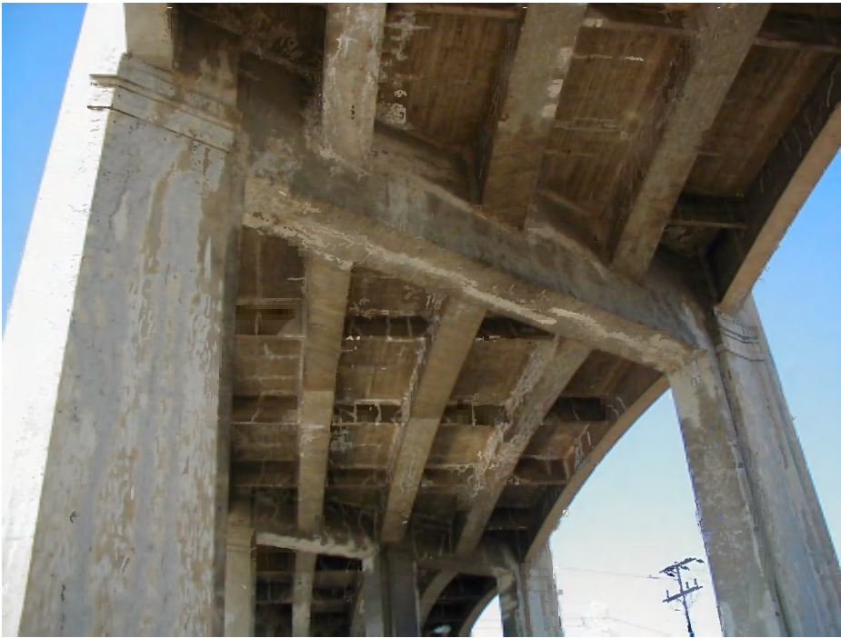
Figure 22: Overall condition of typical bays at the most severely deteriorated sections of the bridge between Bents 12 and 30.
