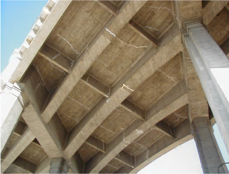
Figure 24: Typical conditions of girders and deck soffit at east end of viaduct between roughly Bents 31 through 39.
