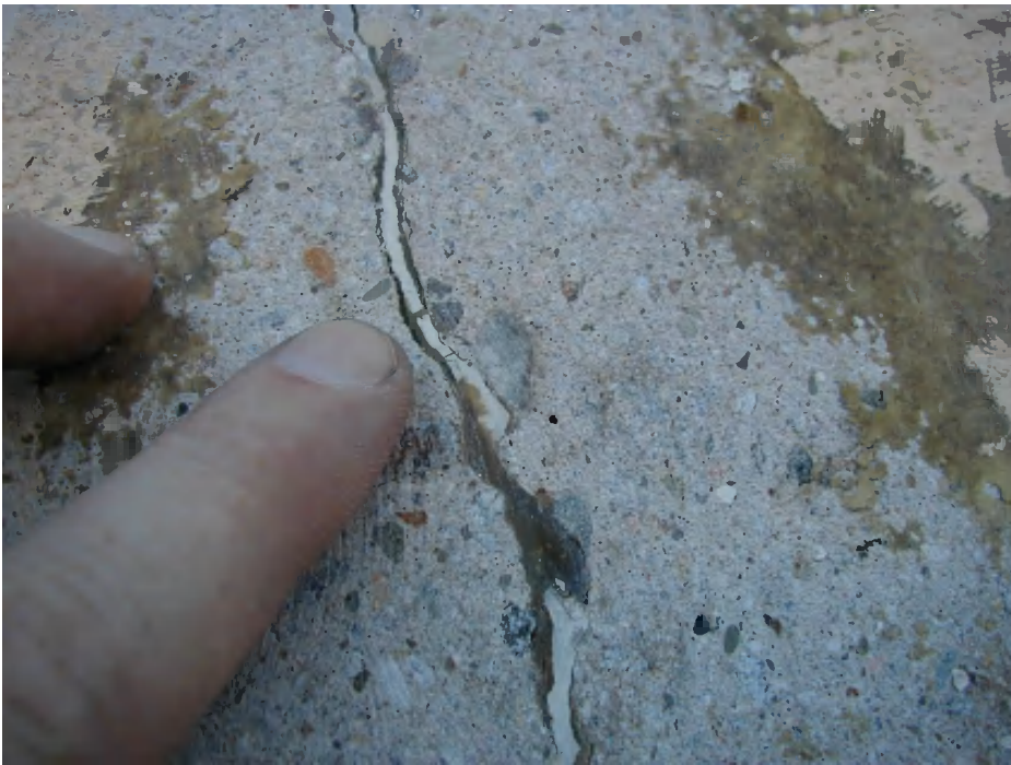
Figure 27: Crack at surface of column with two generations (colors) of epoxy injection and the crack has reopened.
