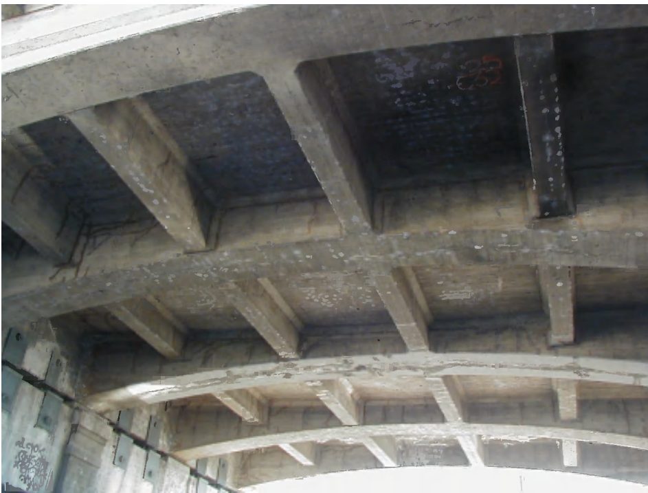
Figure 23: Typical condition of girders and deck soffit at west end of viaduct.
