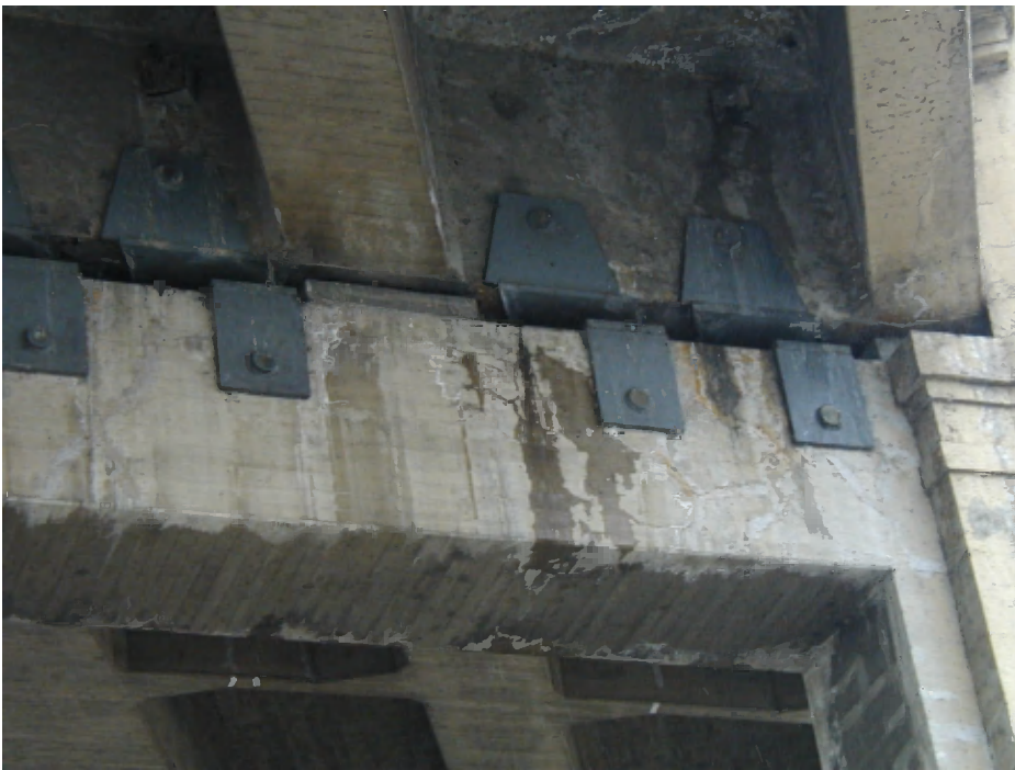
Figure 25: Leaking joint in deck deposits water on top of bent cap. Water migrates into cracks at top of member and emerges through cracks in the face.
