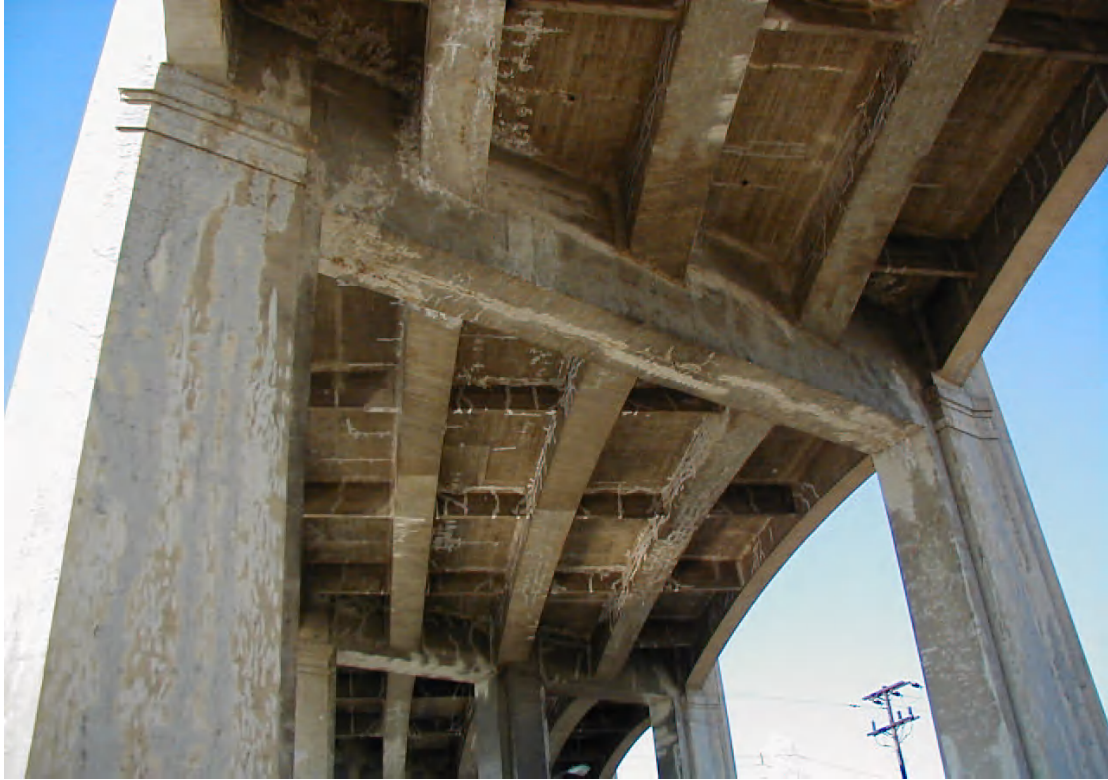
Figure F.10. Typical cracking pattern in bent caps and girders
