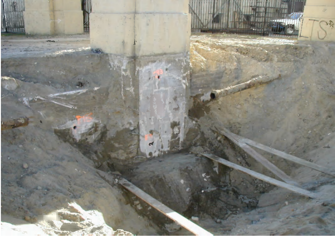
Figure F.14. Cracks in column below ground level
