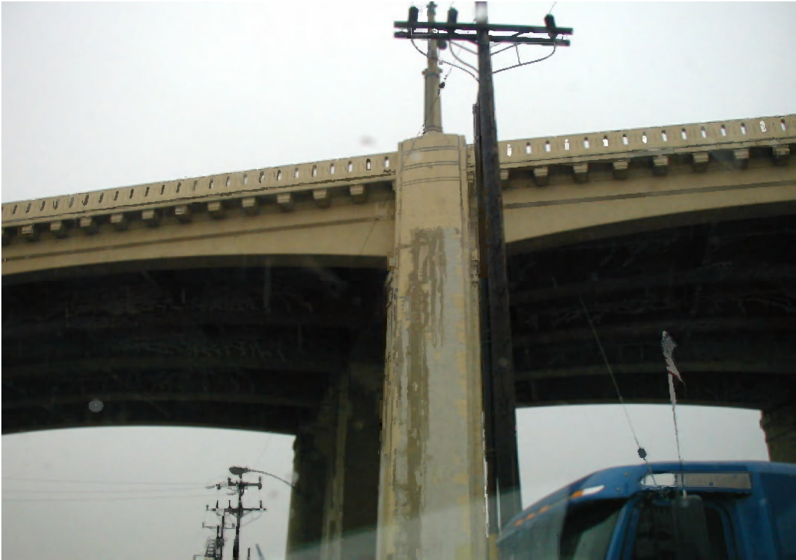
Figure F.16. Water leaking from a typical horizontal column crack at bent cap
