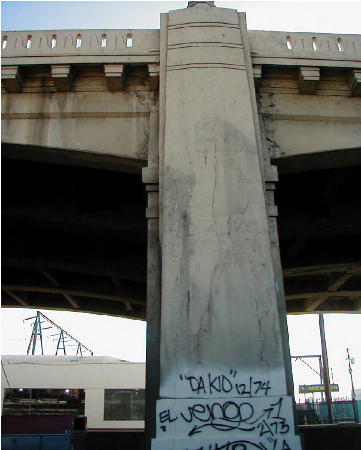
Figure F.7. Typical cracking on outside face of columns and superstructure girders
