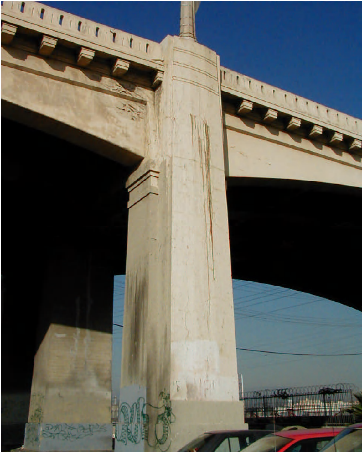
Figure F.9. Typical horizontal cracks in column at level of bent cap
