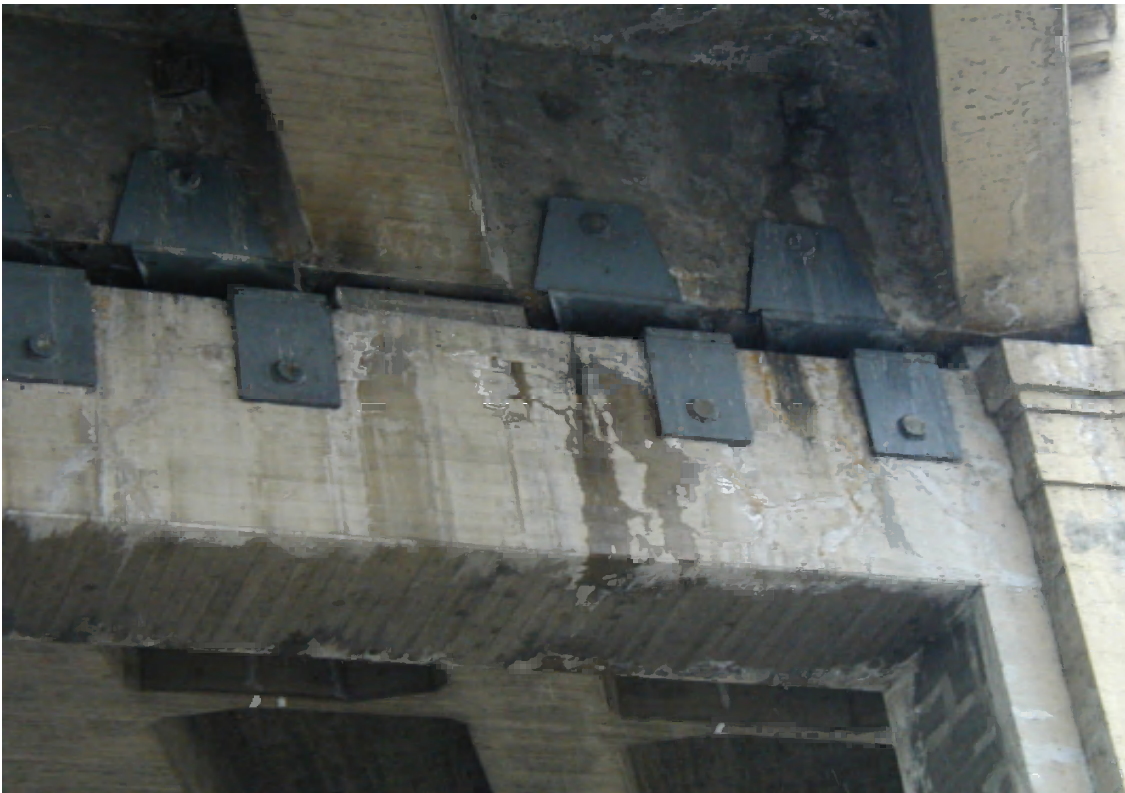
Figure F.15. Water leaking from the deck at an expansion joint
