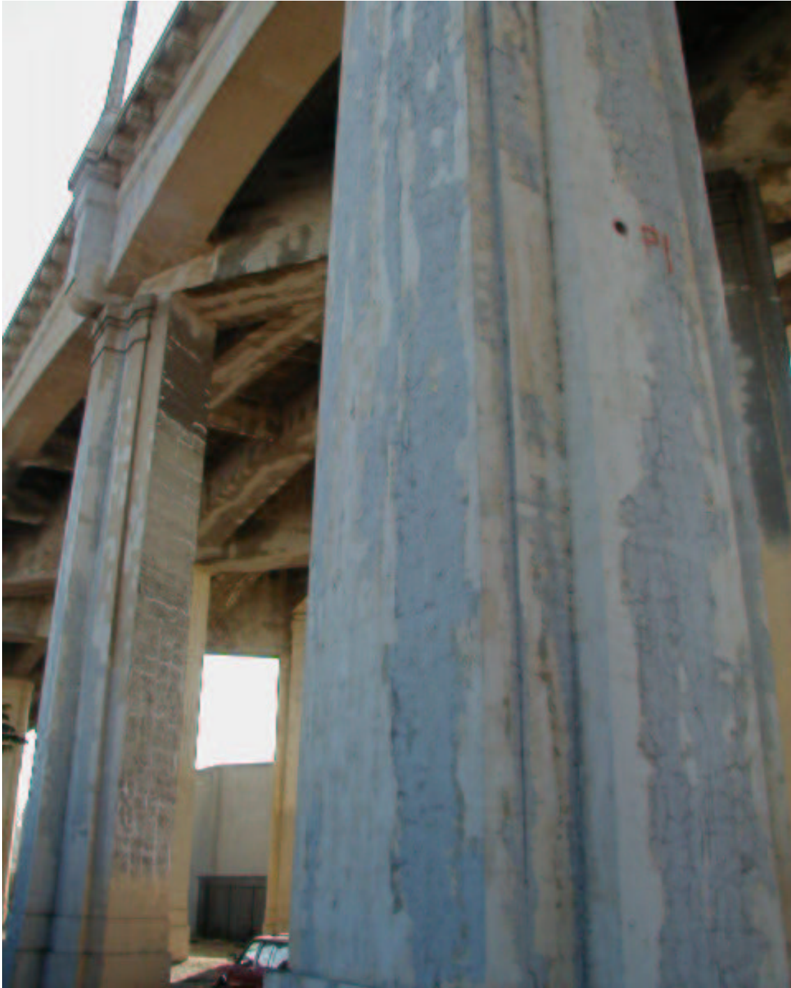
Figure F.8. Typical condition of columns in the east approach spans
