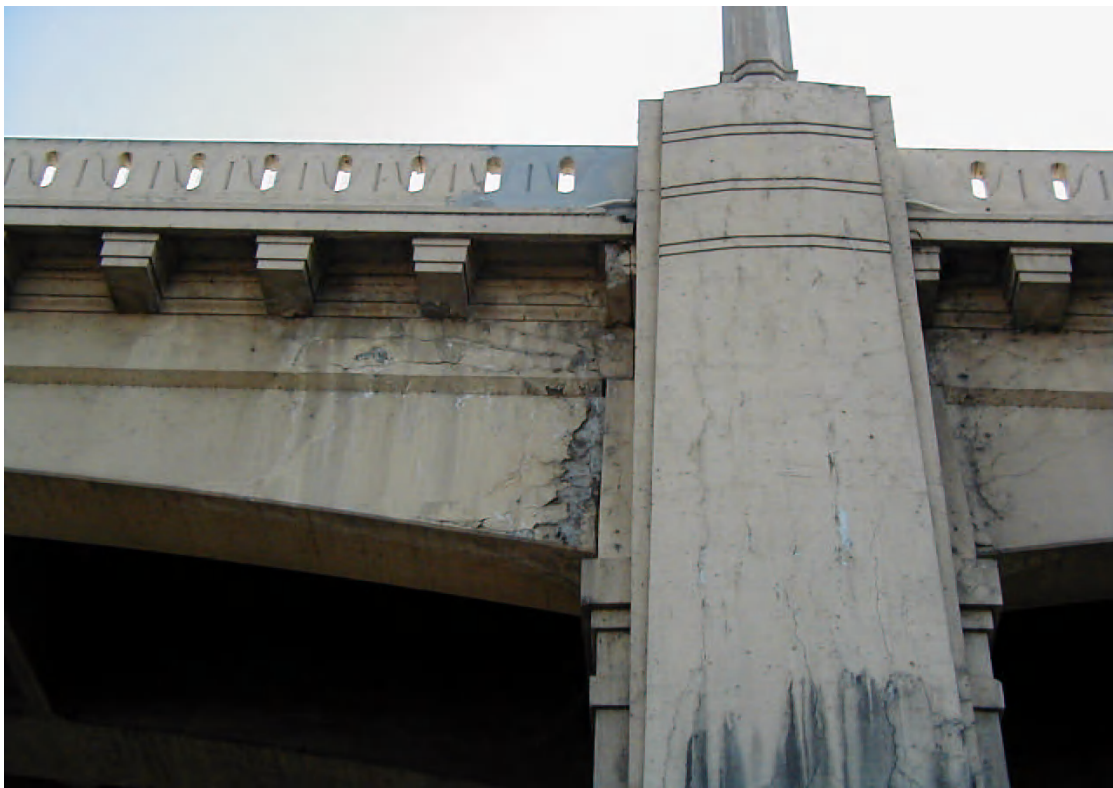
Figure F.11. Cracking in webs of superstructure longitudinal girders
