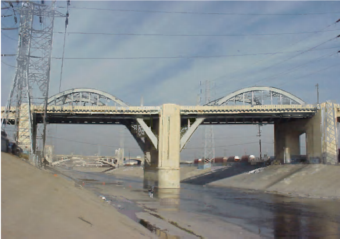
Figure F.3. View of the arch spans over the Los Angeles River looking north
