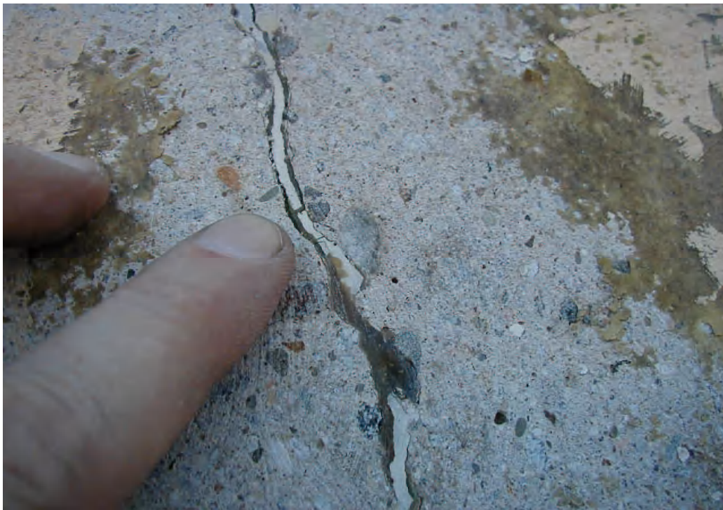
Figure F.13. Reopened crack at surface of column with two generations (colors) of epoxy injection
