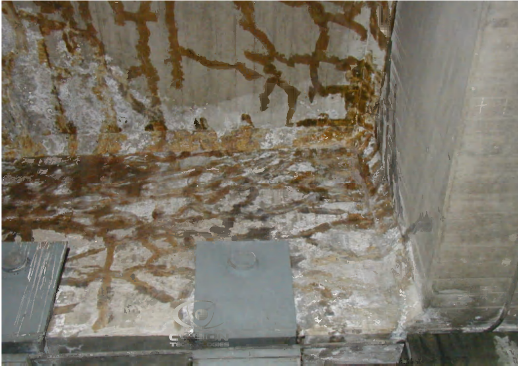
Figure F.12. Severe cracking in bent cap and deck soffit
