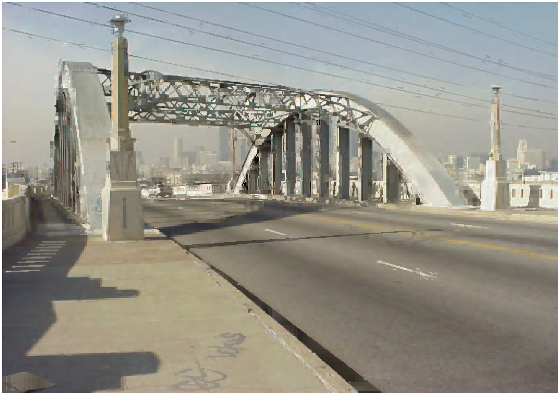
Figure F.4. View of the steel arches from the deck level looking west
